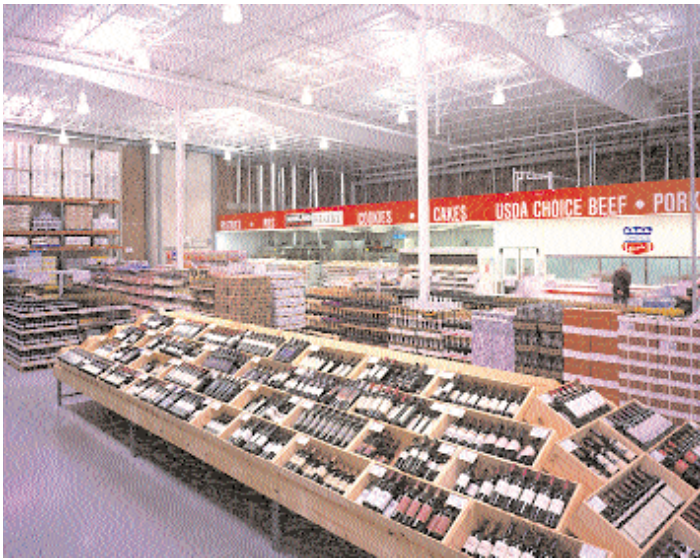
Skylights provide uniform illumination and add highlights in this wholesale store. Note the white ceiling.
